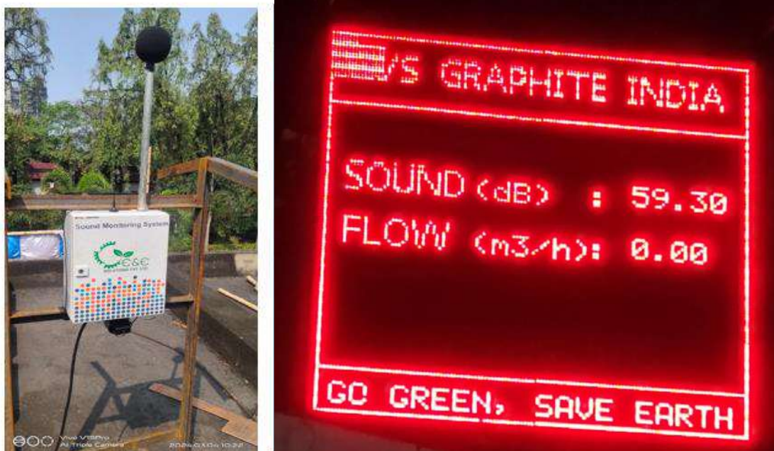
For EC compliance Ambient Noise level Monitoring Station Installed – Commissioning is in process
